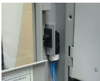
Door Switch in Access Level 1
