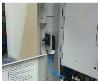
Door Switch in Access Level 2
